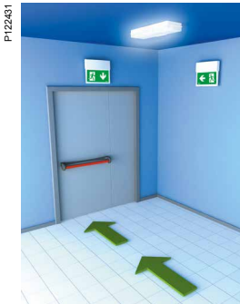
At the safety exits and depending on where the safety signs are installed.
